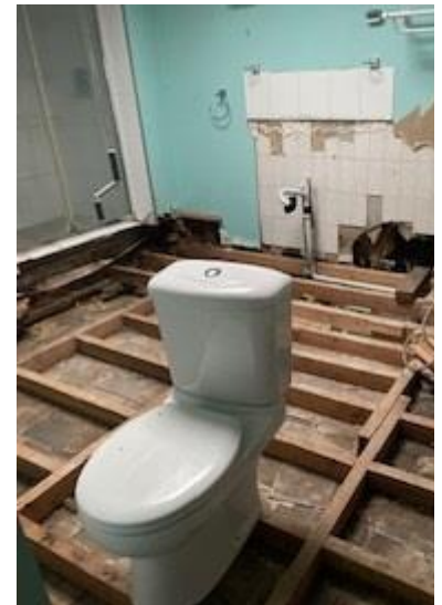
Right: Bathroom floor removed due to damage from flood water at 113
