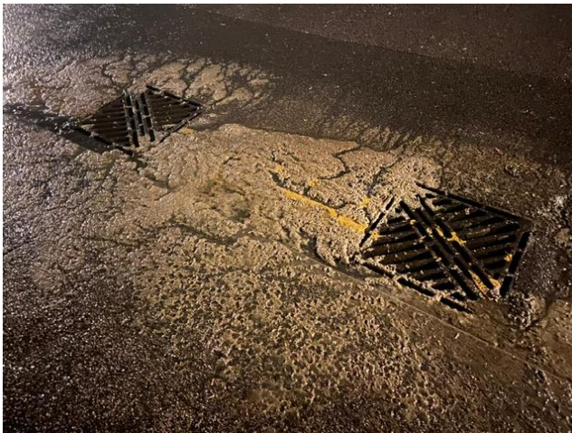
Left: Sewage outside 132 and 134a that spilled onto the properties
